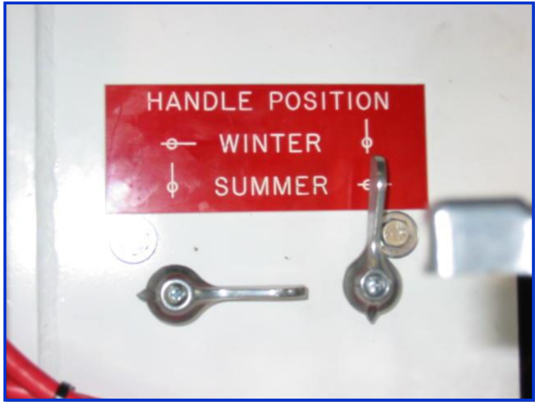
LUBRICATOR HEATER CONTROL VALVE
