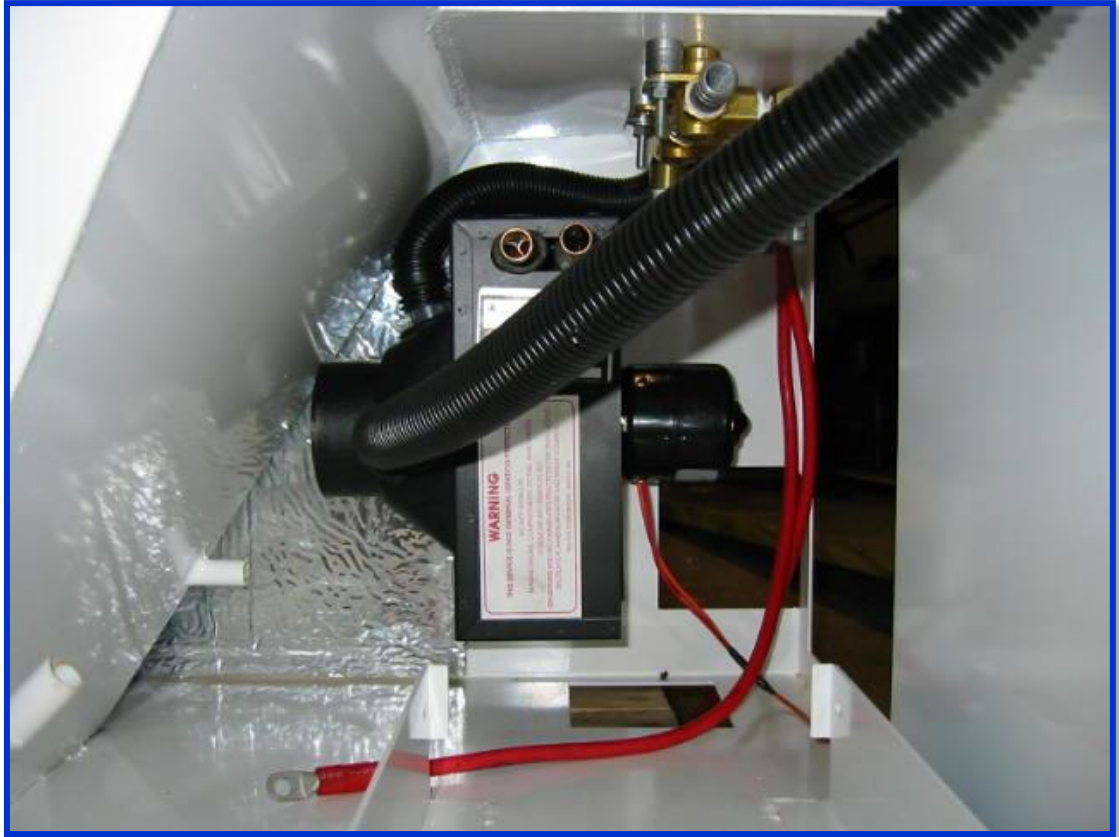
LUBRICATOR HOT WATER HEATER
